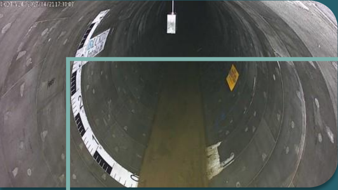
Non - contact discharge measurement (SQ- flowmeter) in a drainage and stormwater tunnel, Hong Kong 非接触式流量测量 (SQ流量 计), 香港排水与暴雨工程涵洞
